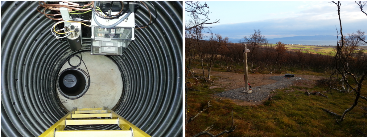
Figure 5.3: Pictures from the broadband station VADS in North-eastern Norway, installed in 2016.
